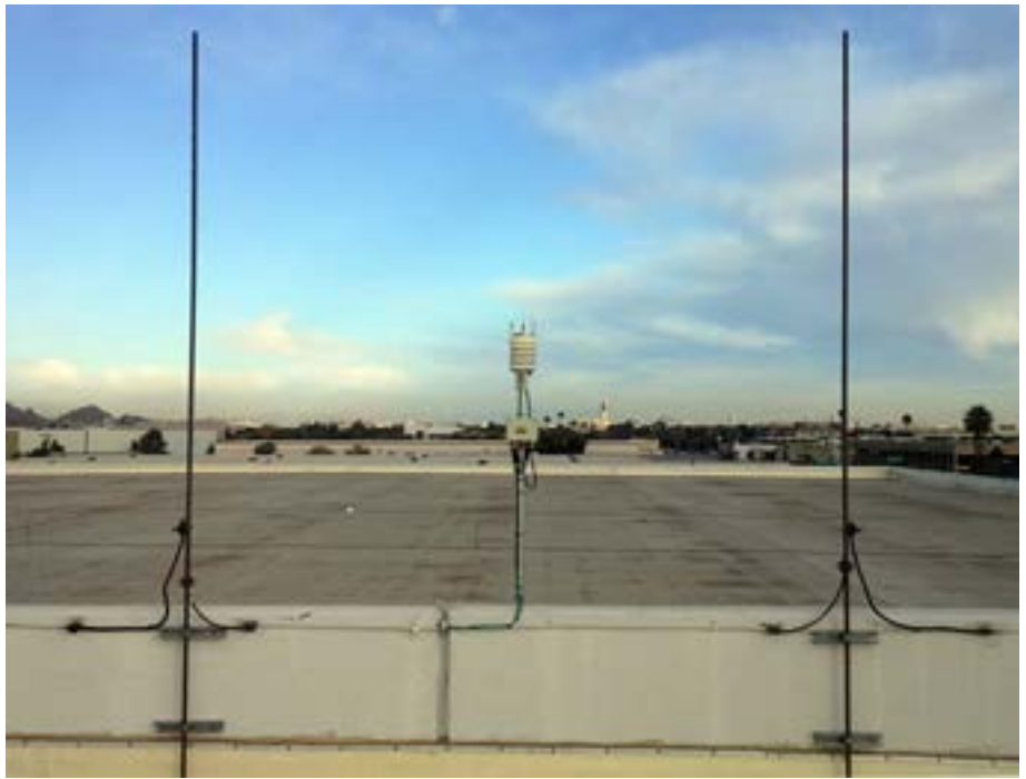
GoDaddy's Orion Weather Station installation on the roof of their Phoenix data center with lightning rods on either side to help protect the sensor.
