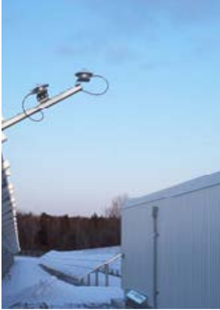
This Solar 1 Weather Station installation shows two radiation sensors, one at plane of array and one at GHI, as well as the Orion weather sensor module on the mast at right. Photo courtesy of Industrial Electrical Contactors Ltd.
