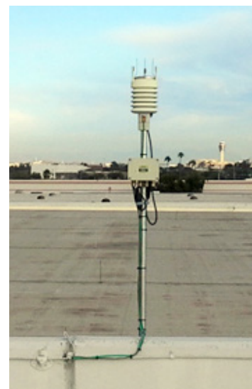
GoDaddy's Orion Weather Station installation in Arizona
